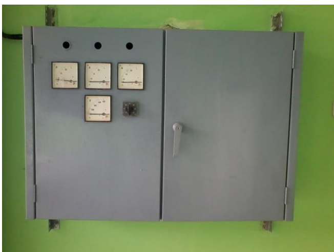
Gbr.19 Panel Listrik
