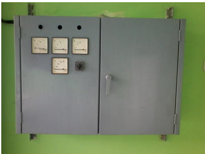
Gbr.19 Panel Listrik
